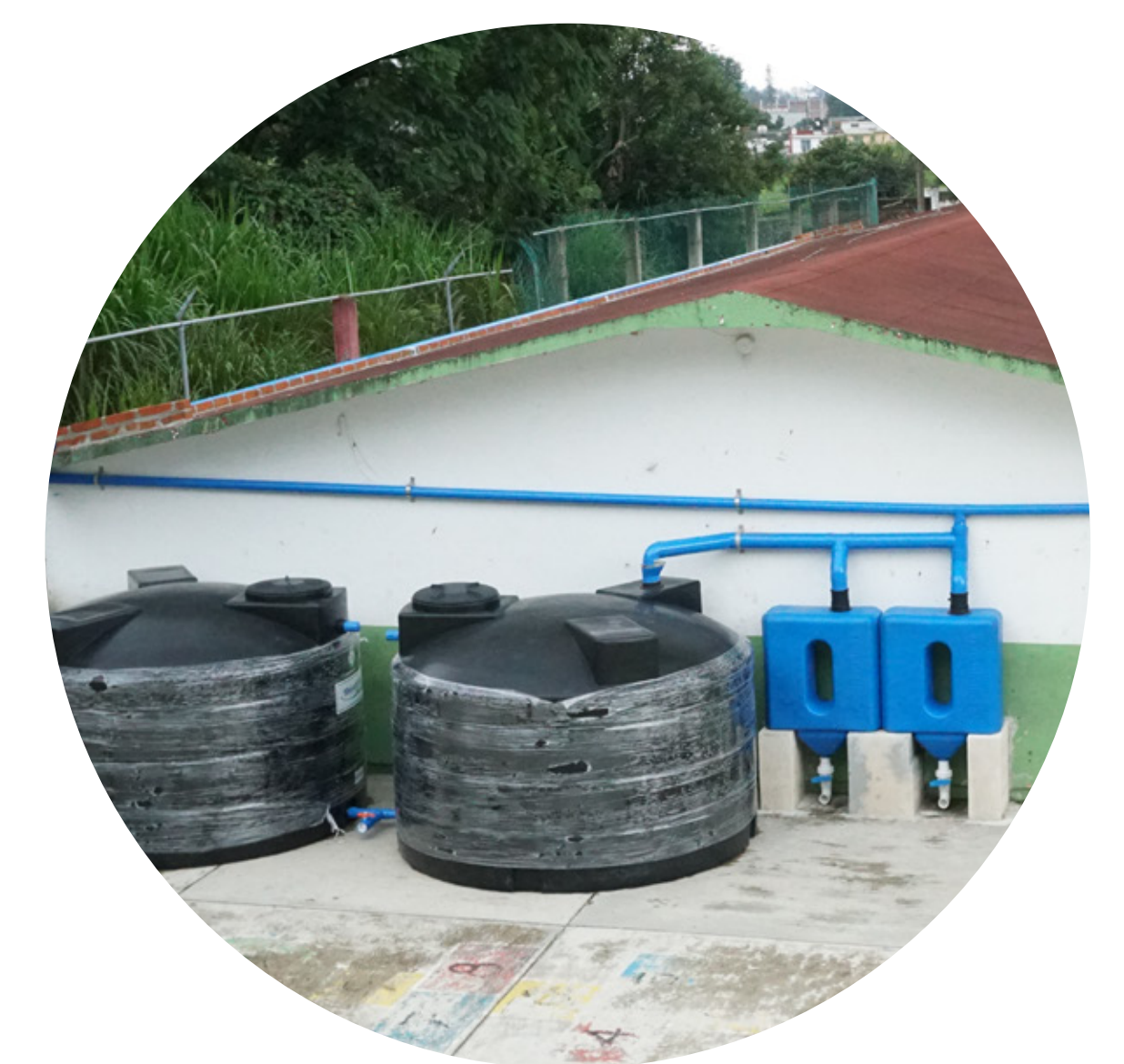
Rainwater Harvesting System
